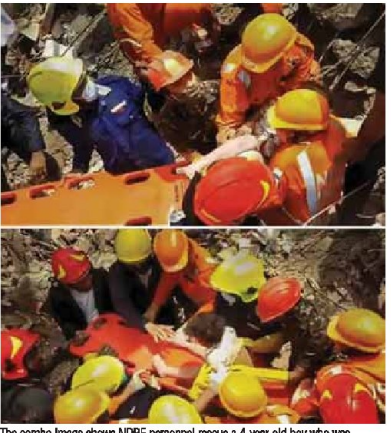
The combo image shows NDRF personnel rescue a 4-year old boy who was trapped under the debris at the building collapse site in Mahad, Raigad
