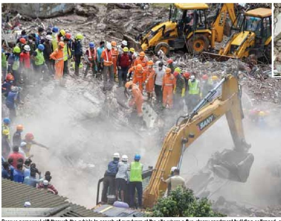
Rescue personnel sift through the rubble in search of survivors at the site where a five-storey apartment building collapsed...
